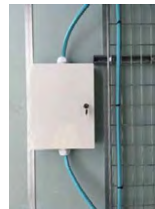
FIBRE OPTIC BREAKOUT BOX INSTALLED WITHIN TENANT'S RISER
