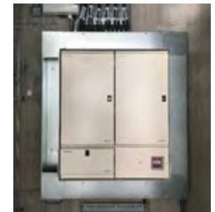
LIGHTING & POWER DISTRIBUTION BOARDS
